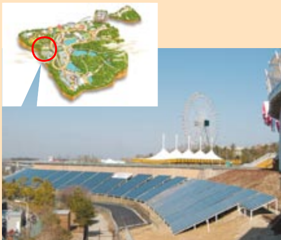
Kyocera's solar modules of 150m in overall length installed at the EXPO site
