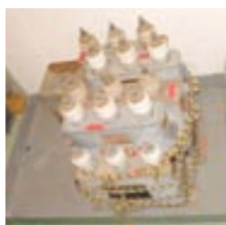
PCB waste storage condition
