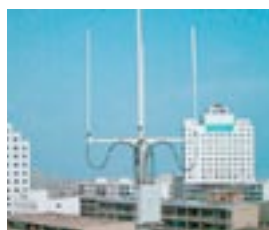
Base Station for Wireless Local Loop
