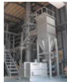
Activated carbon adsorption facility for prevention of dioxins
