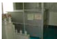
PCB waste storage condition
