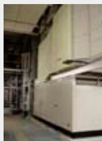
Gas turbine co-generation system
