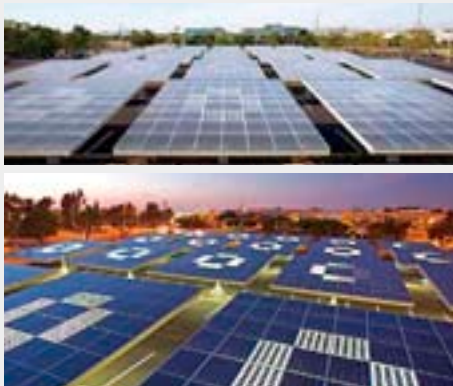
<Solar Trees in Parking Lot: "Solar-Grove">
