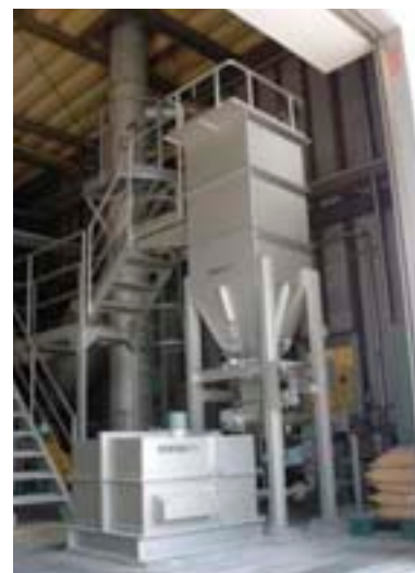
Activated carbon adsorption facility for prevention of dioxins
