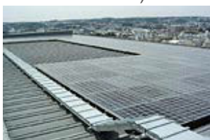
■ Yokohama Office (58kW) (introduced in FY2012)
