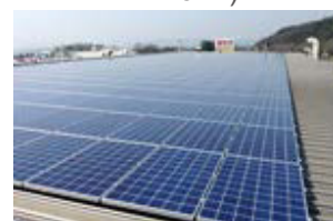
■ Shiga Gamo Plant (491kW) (introduced in FY2011 and expanded in FY2014)
