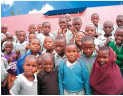
Solar modules installed at a school (Uganda)
