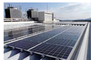
■ Kyocera Document Solutions Inc. Tamaki Plant (50kW) (introduced in FY2011)
