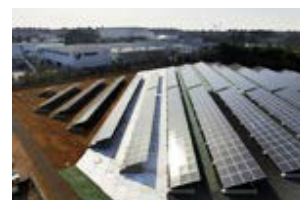
■ Chiba Sakura Plant (493kW) (introduced in FY1985 and expanded in FY2014)
