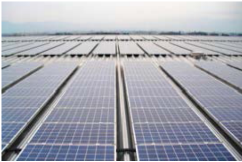
Solar power generating system installed on the plant roof (Shiga Yasu Plant)
