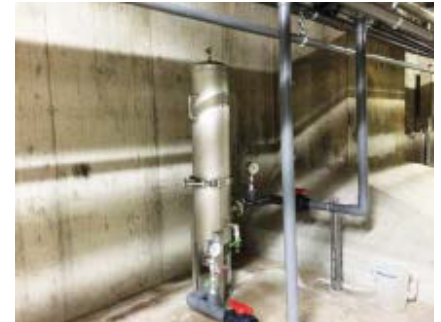
Wastewater Recycling Equipment
