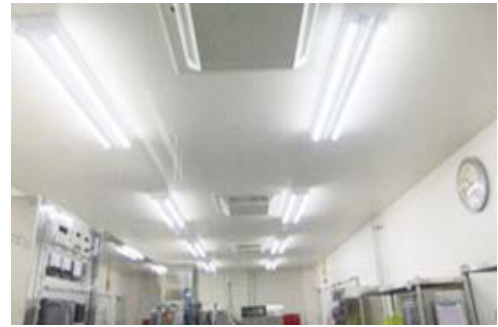
LED lights installed in the clean room (Kagoshima Hayato Plant)
