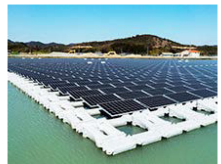
Floating solar power plant in Hyogo Prefecture (Japan)
