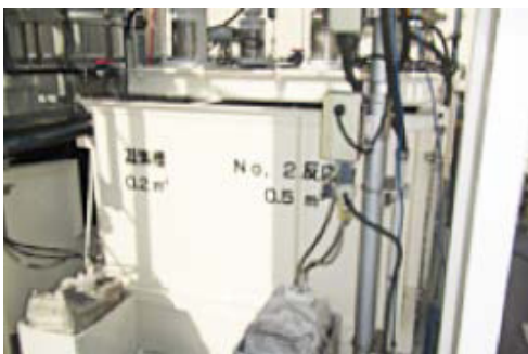
Grinding wastewater treatment equipment (Kagoshima Sendai Plant)
