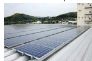
■ Kagoshima Sendai Plant (649kW) (introduced in FY2011 and expanded in FY2014)
