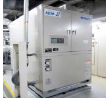
Waste heat recovery chiller
