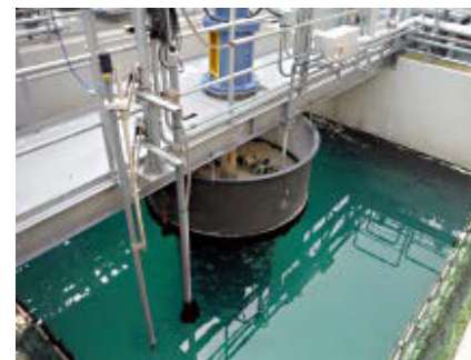
Effluent treatment equipment
