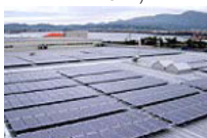
■ Mie Ise Plant (80kW) (introduced in FY2005)
