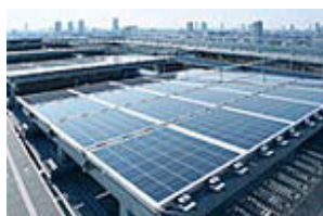
■ Kyocera Document Solutions Inc. Headquarters (12kW) (introduced in FY2008)
