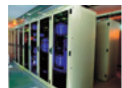
D@TA Center [Kyocera Communication Systems Co., Ltd.]
