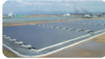
J-POWER Hibikinada Solar Power Plant, Fukuoka Prefecture
