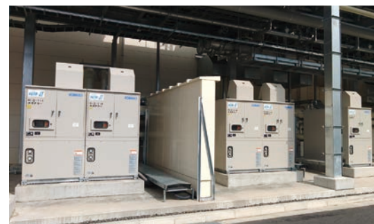
Kyoto Ayabe Plant: Exhaust heat recovery
