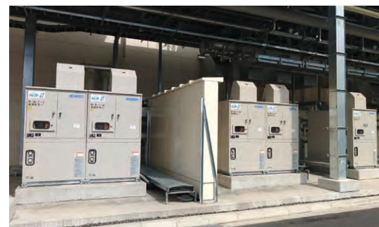
Kyoto Ayabe Plant: Exhaust heat recovery
