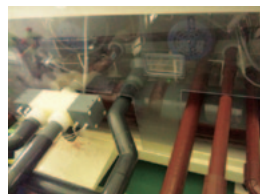
Waste liquid transfer piping
