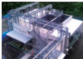
Wastewater treatment plant
