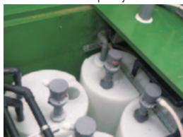
Acid and alkali waste liquid tanks
