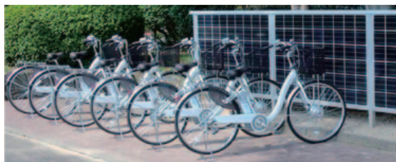
Solar Cycle Station ® installed at Higashi Ohmi City Hall
