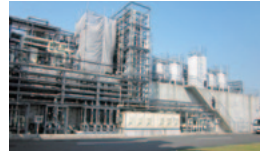
Wastewater treatment plant
