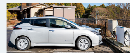
EV charging stations
